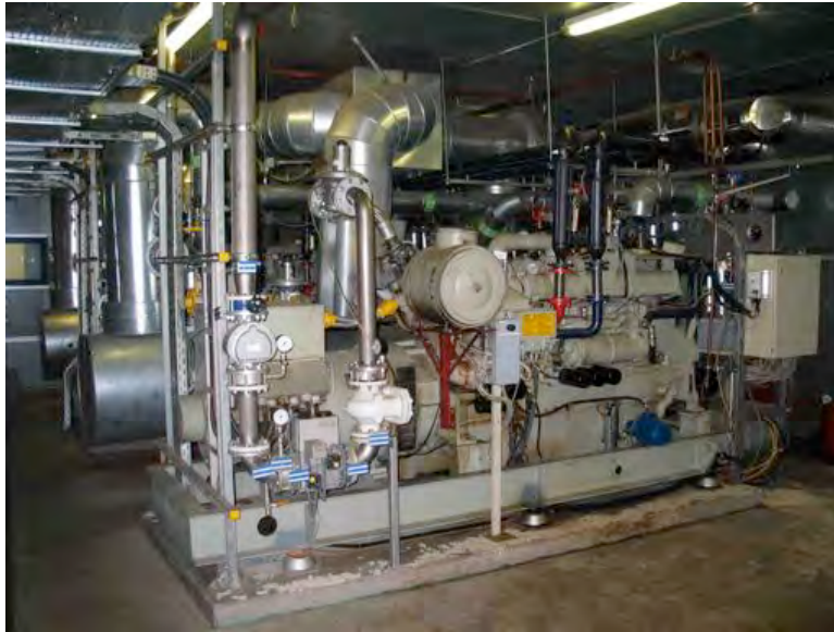
Figure 5.5-7: Unit power station with gas-Otto engine with an electrical output of 375 kW.
