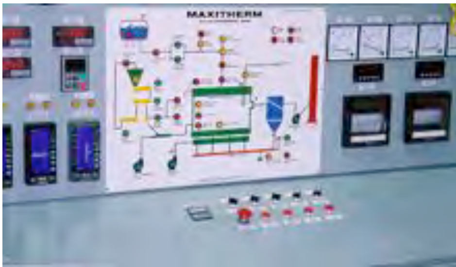
Figure 9.3-3: Boiler control panel
