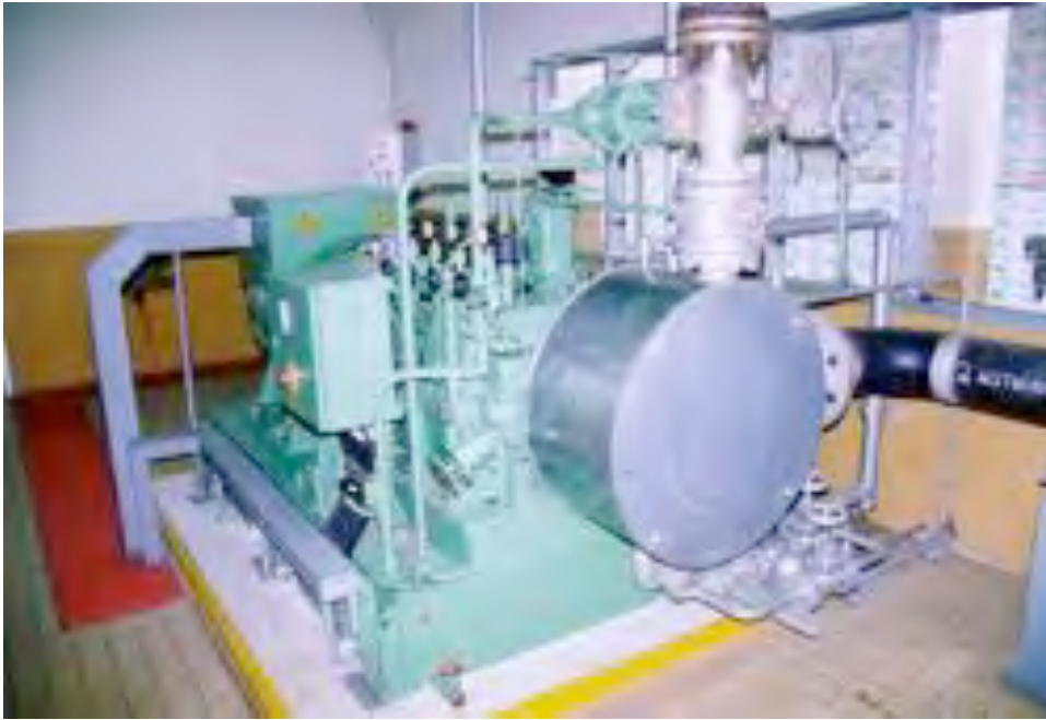
Figure 9.3-2: 250 kW steam turbine
